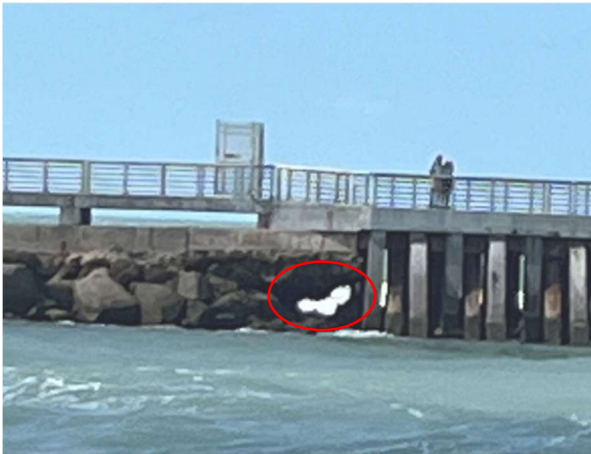
Void below sidewalk to pier transition
