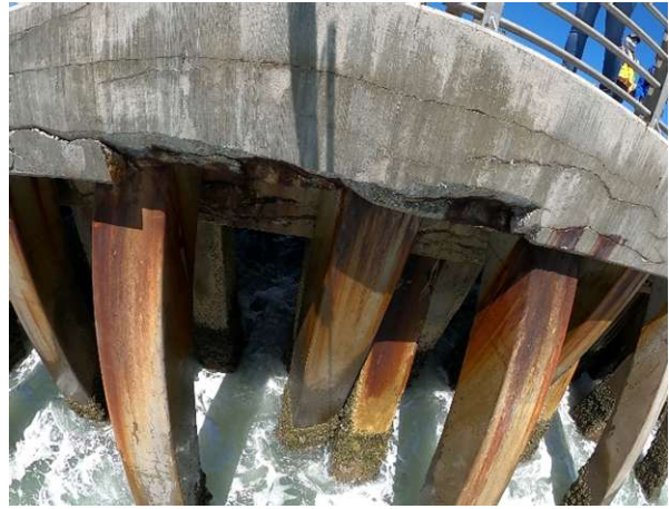
Spalling south face, Bay 30-31
