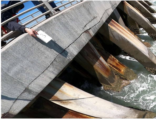
Cracking and delamination south face, Bay 2-4
