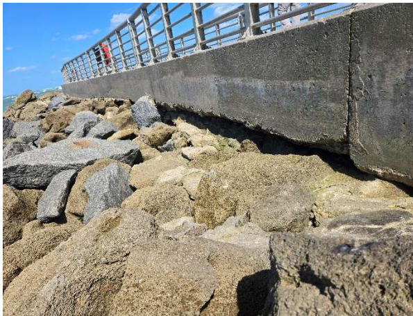
Spalling on bottom of concrete slab and undermining of north face
