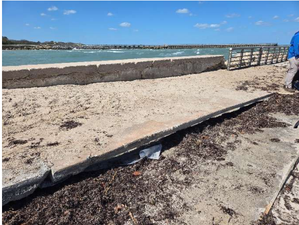
Void underneath sidewalk
