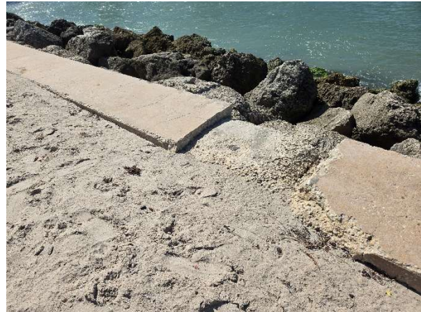
Deteriorated seawall concrete
