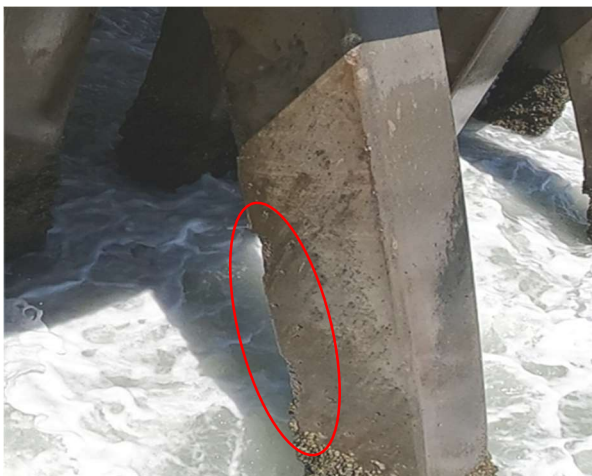
Spall in pile, south face of Bay 56
