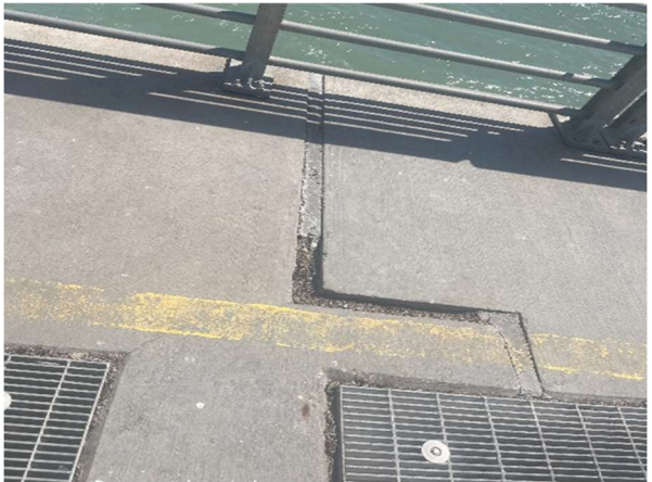
Deteriorated expansion joint material, Bay 18
