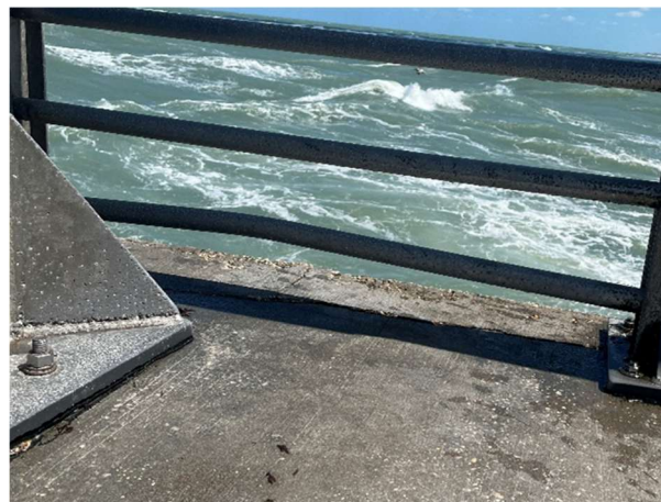
Weather monitoring station base connection
