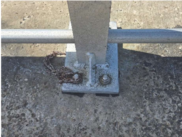
Typical neoprene pad condition
