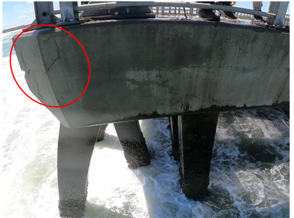
Cracking extreme southeast face
