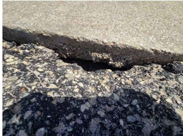
Asphalt void along sidewalk
