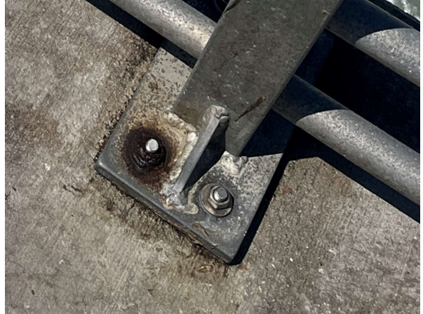
Corrosion of railing base plate & anchor bolts, Bay 37
