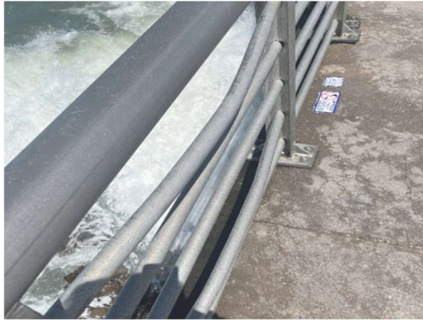
Bent guardrail, Bay 52 North
