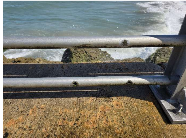
Deterioration of railing member and pitting
