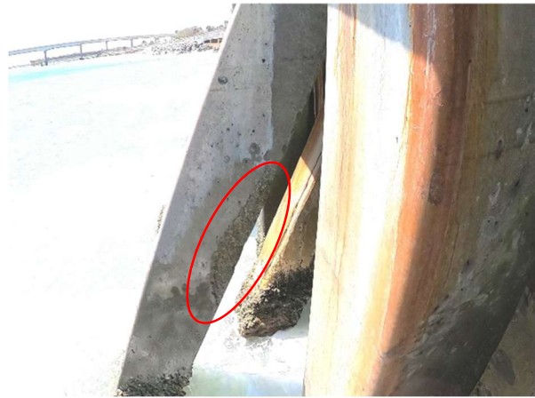
Spall in pile, south face of Bay 5
