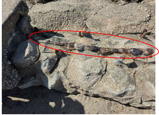
Exposed sheet pile wall with corroded steel
