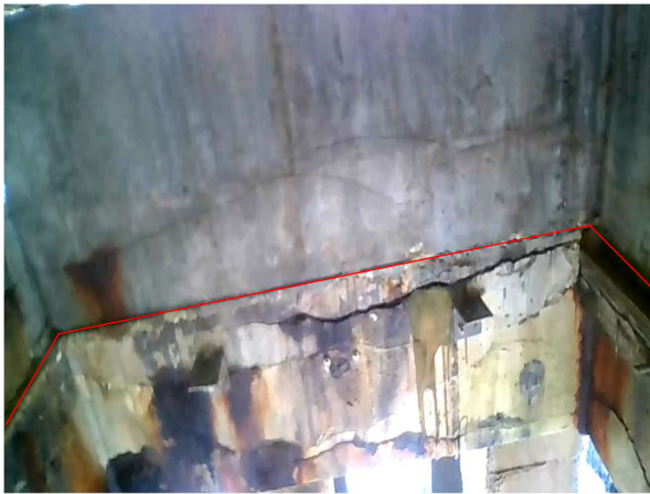
Typical cracks and rust bleeding bay openings
