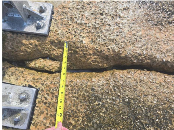
Concrete surface erosion and spalling
