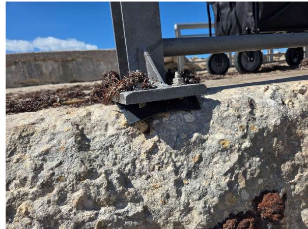
Base plate partially unsupported near west end
