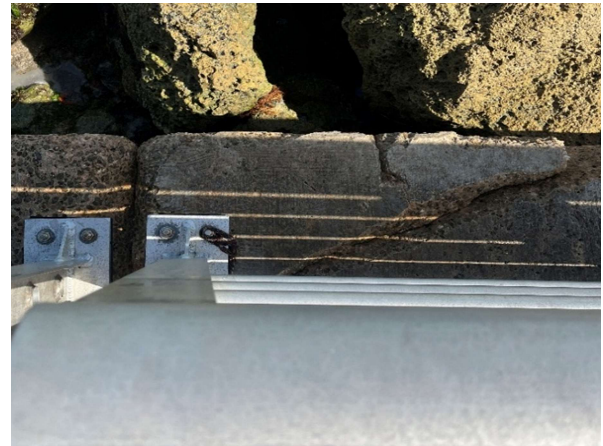
Corner crack in slab at joint
