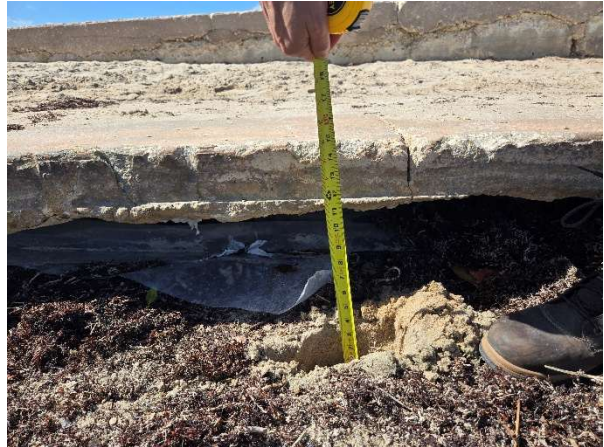
Void underneath sidewalk
