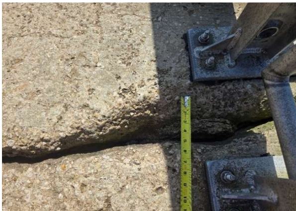
Corner spall in slab at joint
