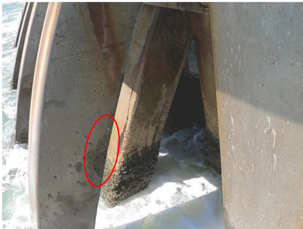
Spall in pile, south face of Bay 6
