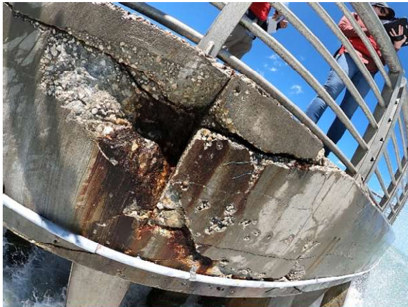
Cracking and heavy spalling south face, Bay 57
