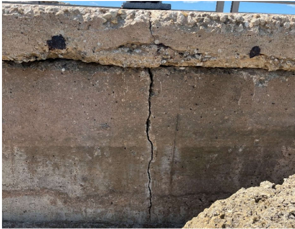
Cracking on pier slab – south face
