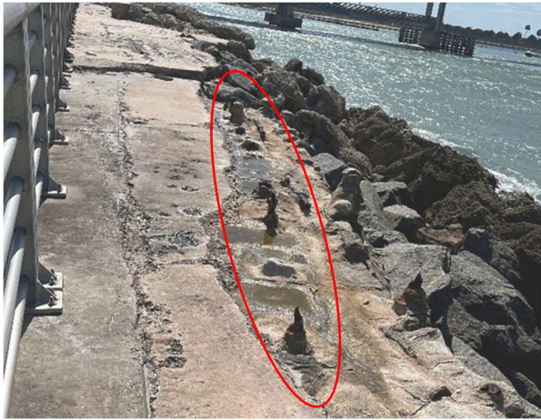
Exposed sheet pile wall with corroded steel
