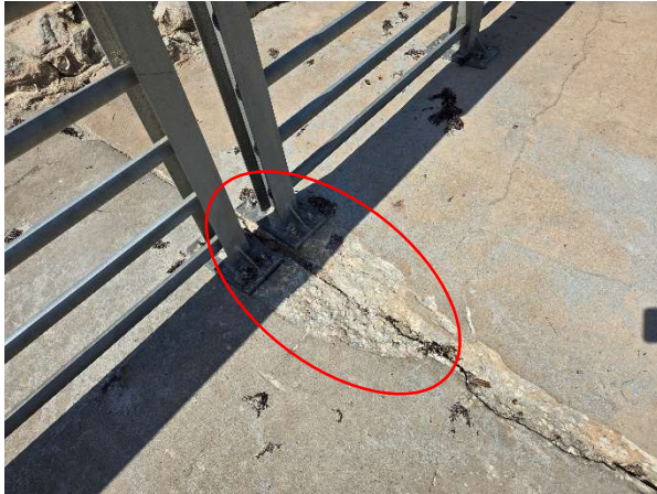
Typical corner spall in slab at joint
