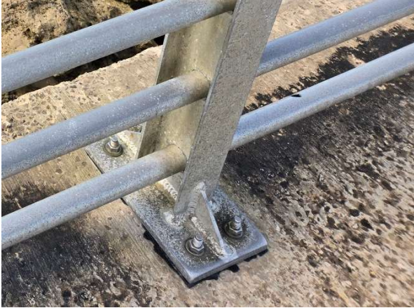
Corrosion of base plate
