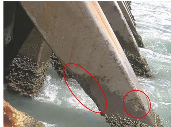
Spall in pile, south face of Bay 38
