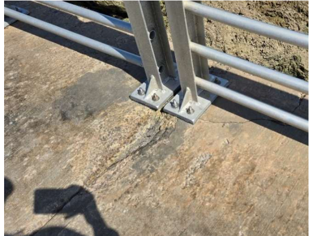
Typical corner spall in slab at joint
