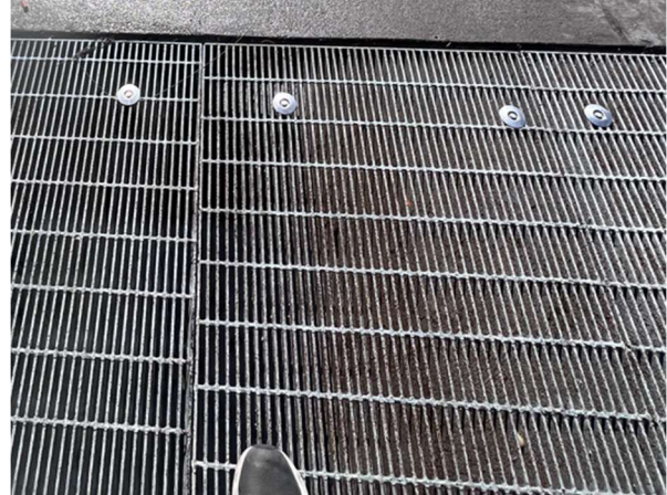
Typical corrosion of steel grating
