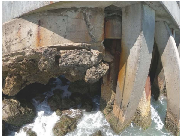
Void below sidewalk to pier transition
