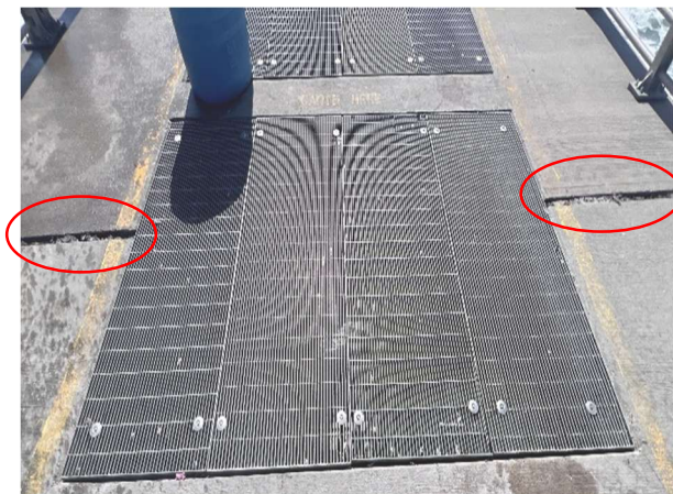
Deteriorated expansion joint material, Bay 37
