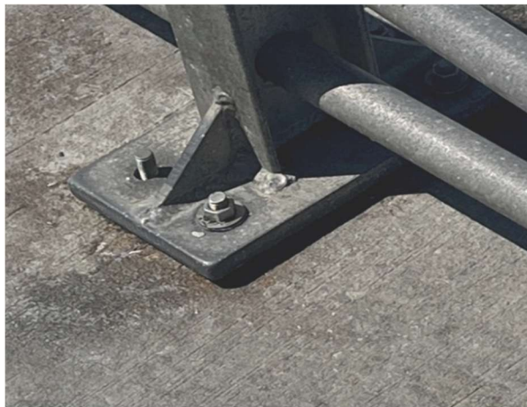
Bolt nut missing on guardrail plate, Bay 37
