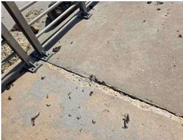
Spall in concrete pier slab
