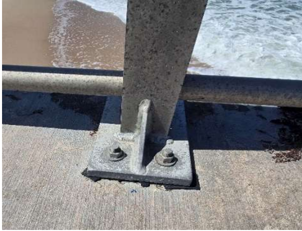
Typical neoprene pad condition
