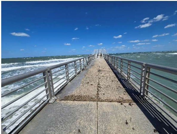
Typical elevated sidewalk surface abrasion
