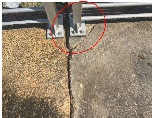
Corner crack in slab at joint
