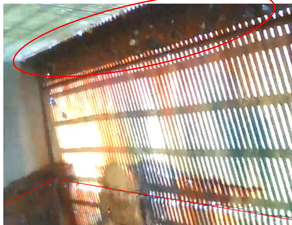
Corroded grating support angle, Bay 16
