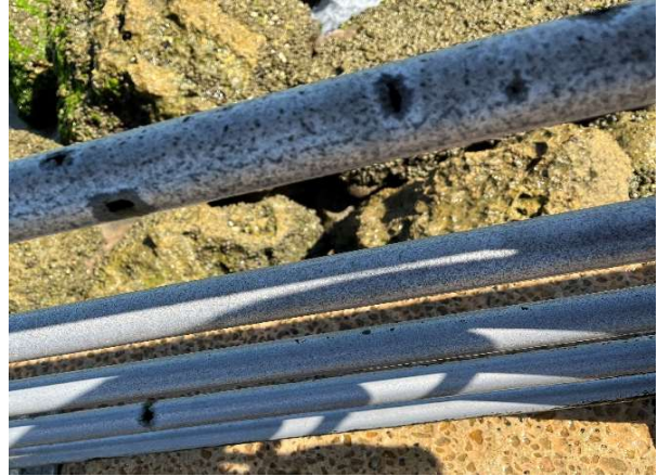
Deterioration of railing member
