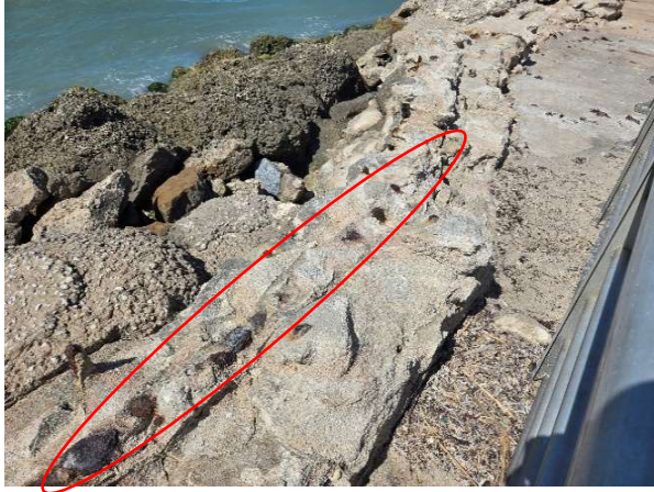
Exposed sheet pile wall with corroded steel
