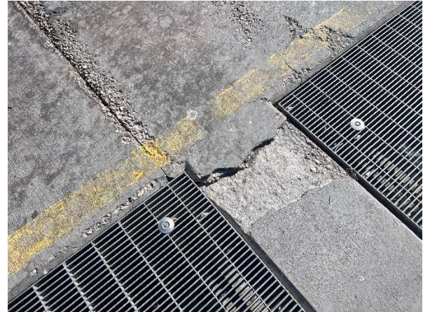
Spall at top of pile cap, Bay 33
