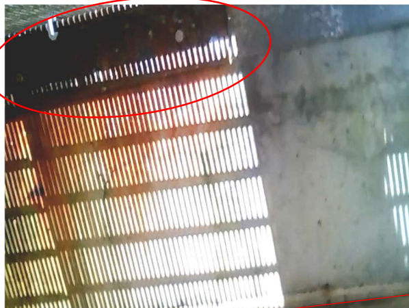
Corroded grating support angle, Bay 6
