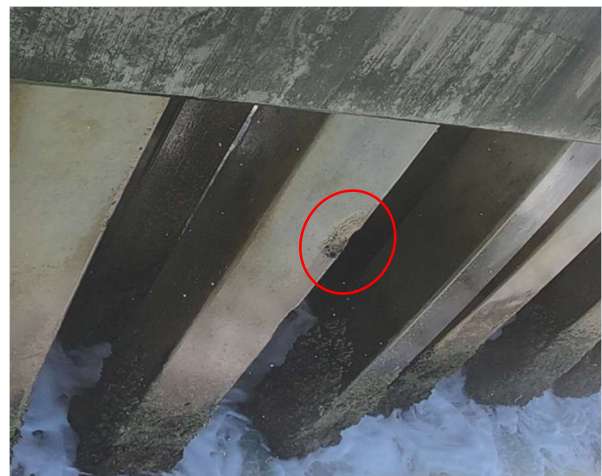
Spall in pile, north face of Bay 59
