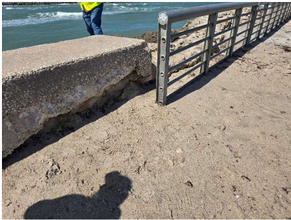
Deteriorated seawall concrete
