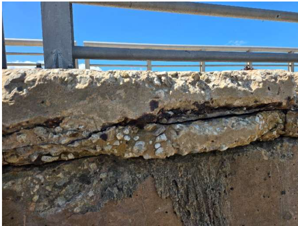
Spalling of concrete slab with exposed reinforcement—south face
