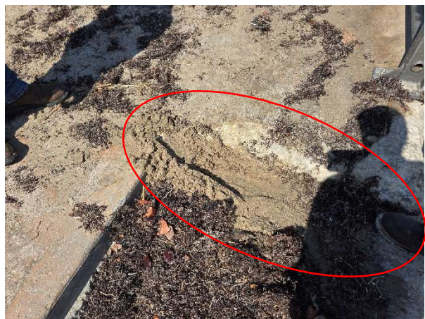
Tripping hazard caused by sand erosion
