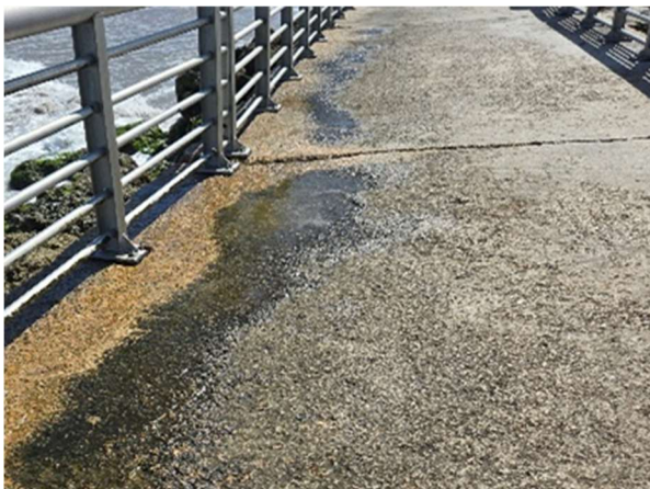
Concrete surface erosion
