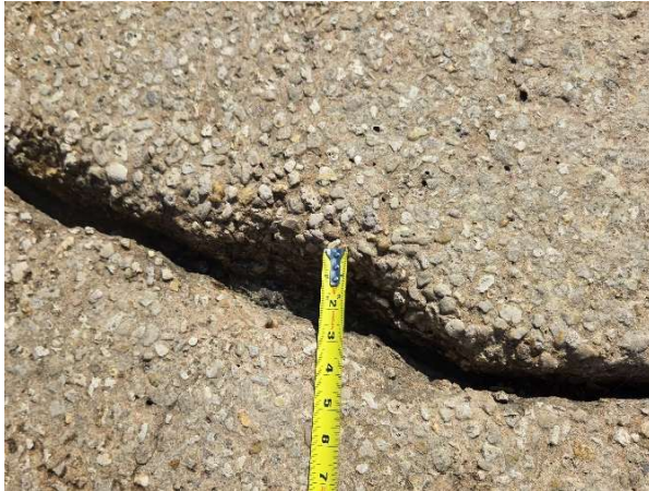
Concrete surface erosion
