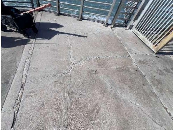
Cracks east of the gate
