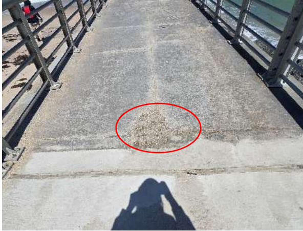
Exposed aggregate at control joints
