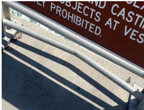
Bent guardrail, Bay 54 South
