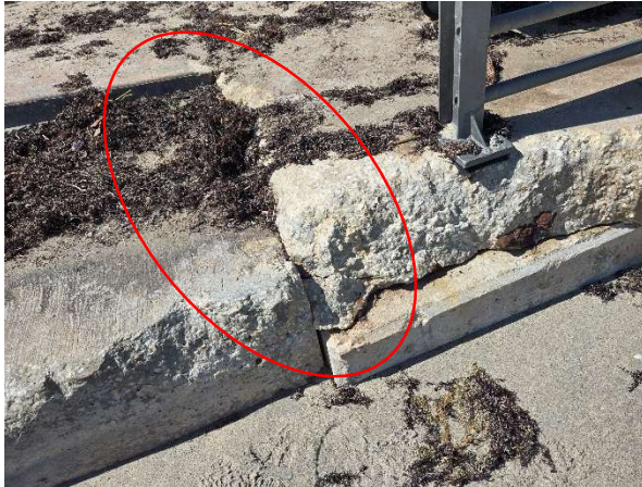
Tripping hazard caused by sand erosion
