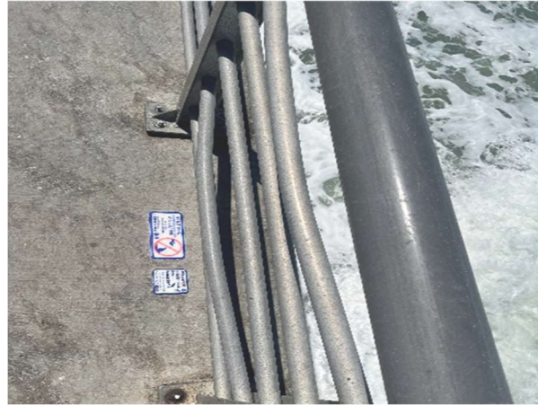
Bent guardrail, Bay 37 South
