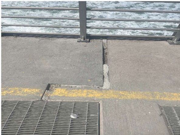
Deteriorated expansion joint material, Bay 18
