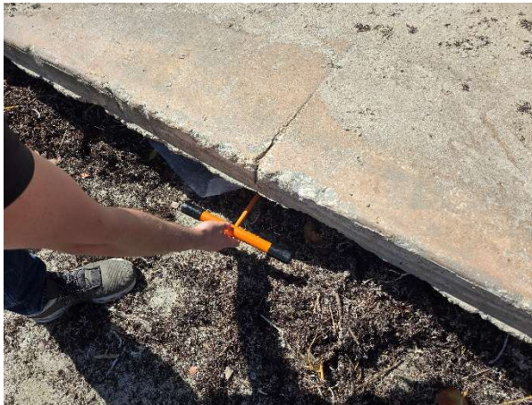
Void underneath sidewalk
