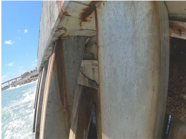
Rust bleeding on pile and pile cap, south face of Bay 6
