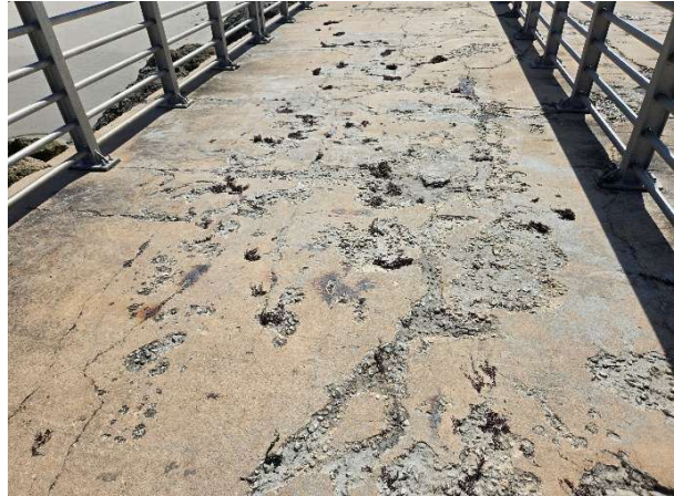
Typical surface erosion
