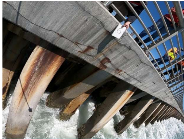
Rust bleed top of pile, south face of Bay 6
