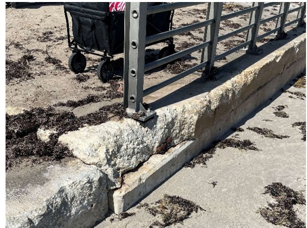
Spalling on concrete pier slab – south face
